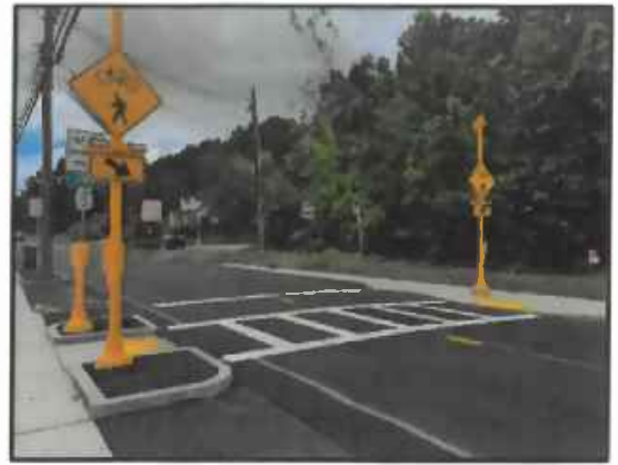
Rapid Flash Beacon - O'Brien's Corner - Springfield St
